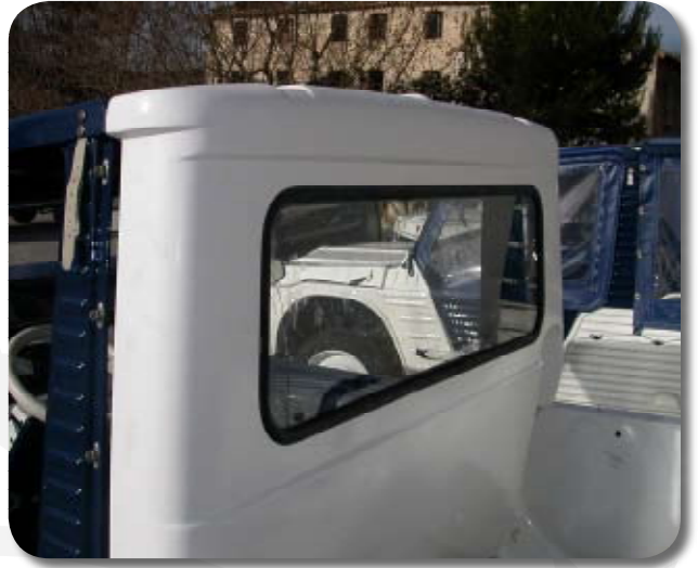
6/ Fit the roof inside the pick up element which is fix for the lower part.
